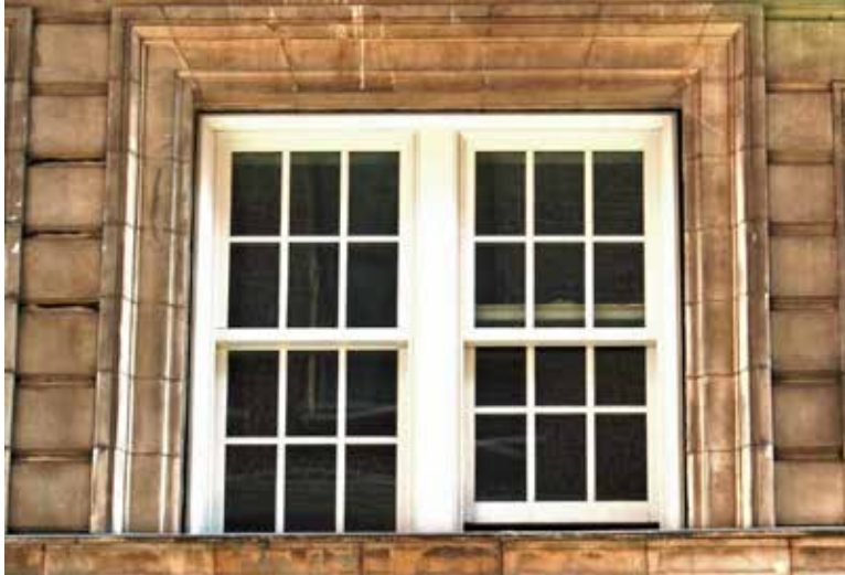
Image: Courtesy of Heritage Consulting Group Aluminum-clad wood windows (pictured) replaced the historic windows of the 1913 Winecoff Hotel in Atlanta.
