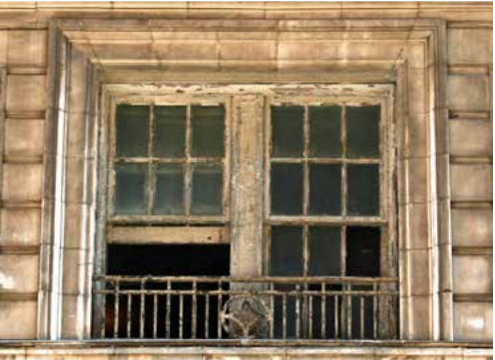
Image: Courtesy of Heritage Consulting Group The original windows of the Winecoff Hotel in Atlanta were in poor condition and needed to be replaced during renovation.
